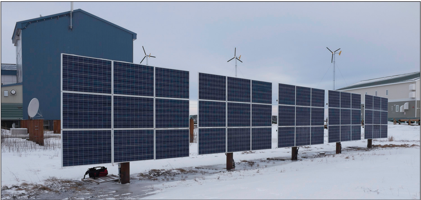
Solar PV array in Bethel. Photo by Gwen Holdmann/ACEP.
