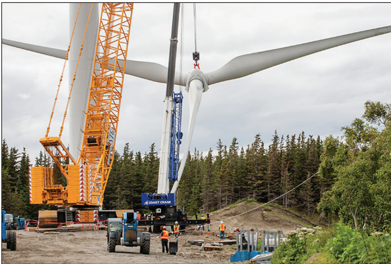
Construction of the Fire Island Wind Farm, developed by Fire Island Wind LLC, which is a wholly owned subsidiary of CIRI Native Corporation. The 17.6 MW project provides power to the Railbelt grid under a long-term power purchase agreement with Chugach Electric Association.
