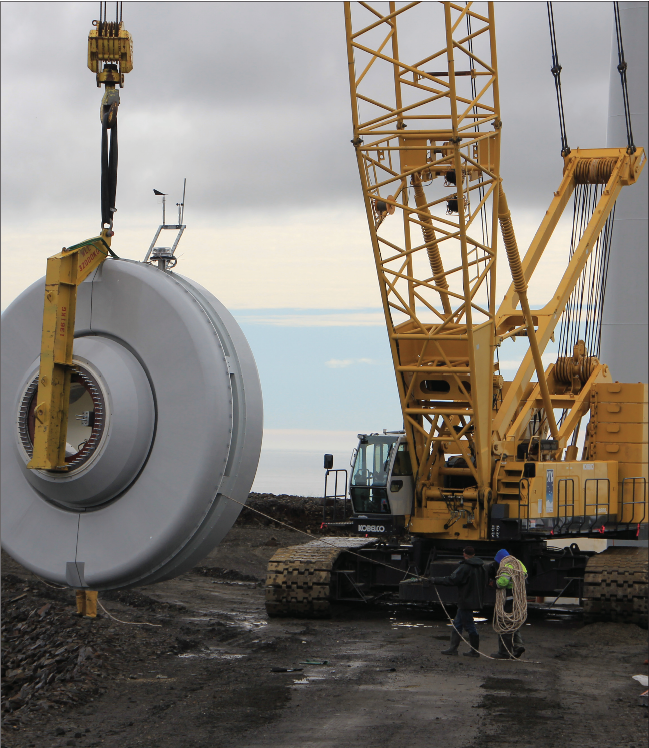
Nacelle of a 900 kW EWT direct drive wind turbine being lifted into position during construction of the second phase of the Banner Wind Peak Farm near Nome. Photo by Gwen Holdmann, ACEP.
