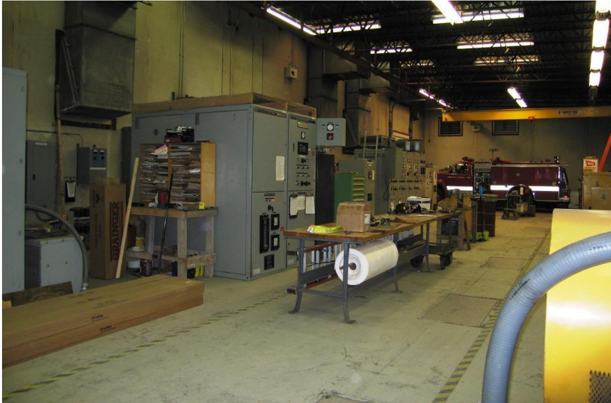
Figure 4: The interior of a power plant in the village of St. Paul in the Pribilof Islands. Source: Photo Credit: Department of Commerce, Community and Economic Development; Division of Community and Regional Affairs' Community Photo Library.
