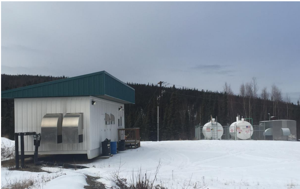
Figure 3: A power plant and fuel tanks in the village of Ruby.
